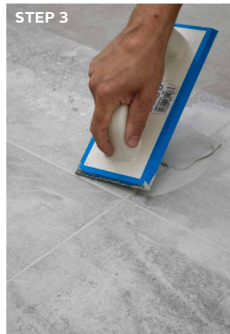
STEP 3 Proceed to grouting a minimum of 3 hours after the start of the adhesive application.
