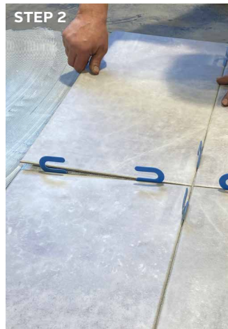
STEP 2 And now apply the tiles using spacers within the next 30 minutes. Take the spacers out within 45-60 minutes and roll the floor.
